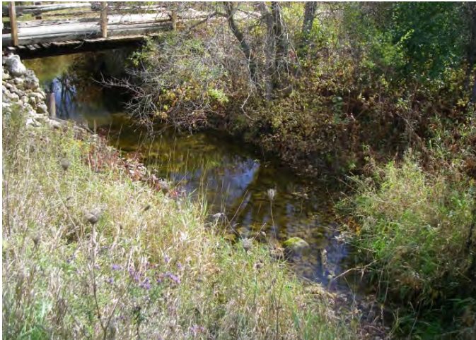
Photo 21: Station 18-3a – No. 21 Drainage Works (Fall 2012) - Facing upstream (southeast) from Concession 8 & 9, showing channel overview.
