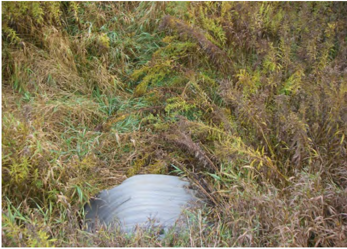
Photo 37: Station 3-2 – Atkinson Drainage Works (Fall 2012) at Concession Road 4 & 5, showing channel definition at culvert.
