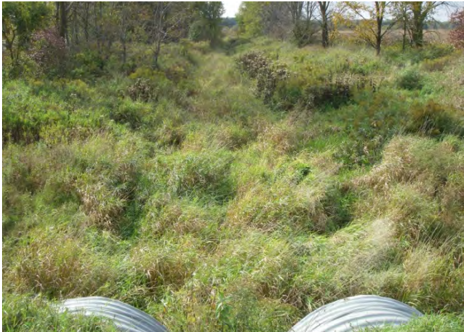
Photo 29: Station 12-4 – No. 7 Drainage Works (Fall 2012) - Facing upstream (west) from Sideroad 27 & 28, showing channel overview and surrounding forest.
