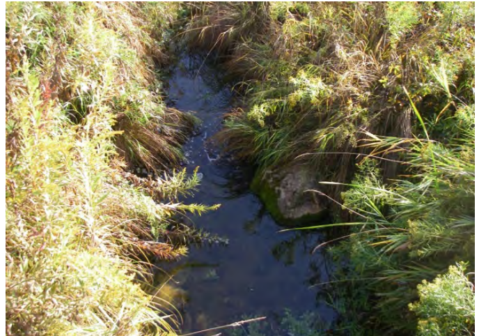
Photo 28: Station 17-1 – Gajtani Drainage Works (Fall 2012) at Sideroad 27 & 28, showing water in channel and bank definition.
