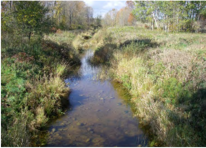
Photo 13: Station 19-1 – No. 16 Drainage Works (Fall 2012) - Facing upstream (west) from Sideroad 24 & 25, showing channel overview.
